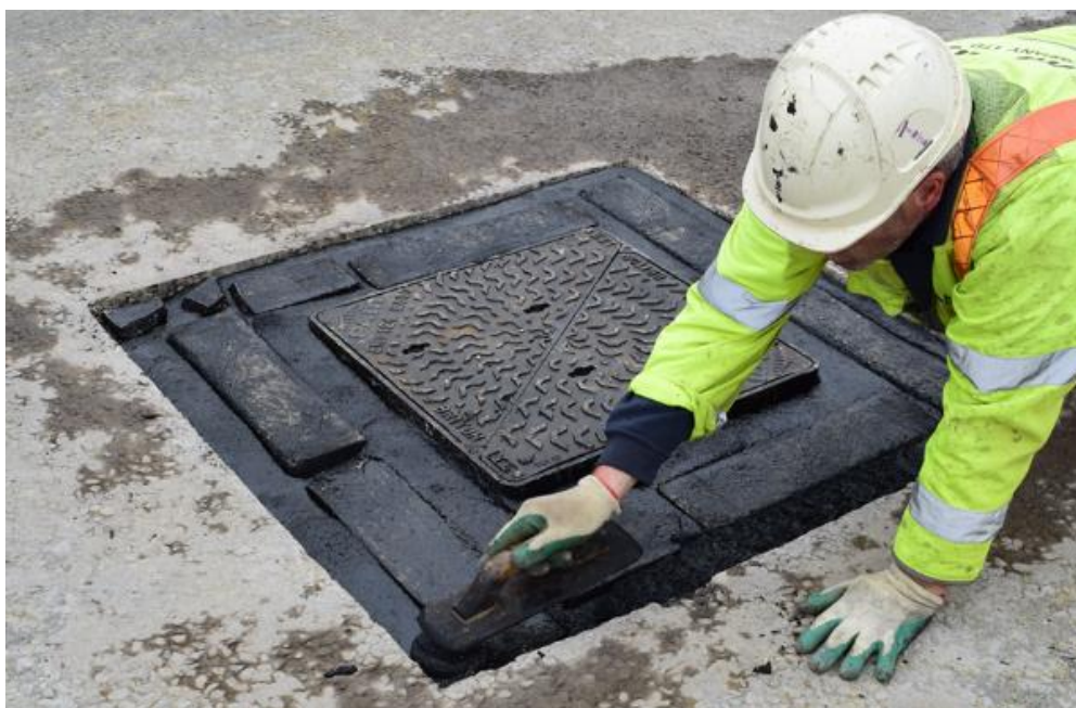
Figure 550- 10 Alternative A – Permitted: Placing of Hot Surfacing (Mastic Blocks) onto Mastic Base
